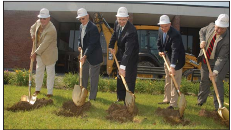
CEREMONIAL DIG - In attendance of the ground breaking ceremony for the Robert R. Jorgensen Athletic Center were: from left - MVCC alumnus Michael Briggs, Robert Jorgensen, President Randall VanWagoner, Oneida County Executive Anthony Picente, and Board of Trustees Chair William Calli, Jr.
